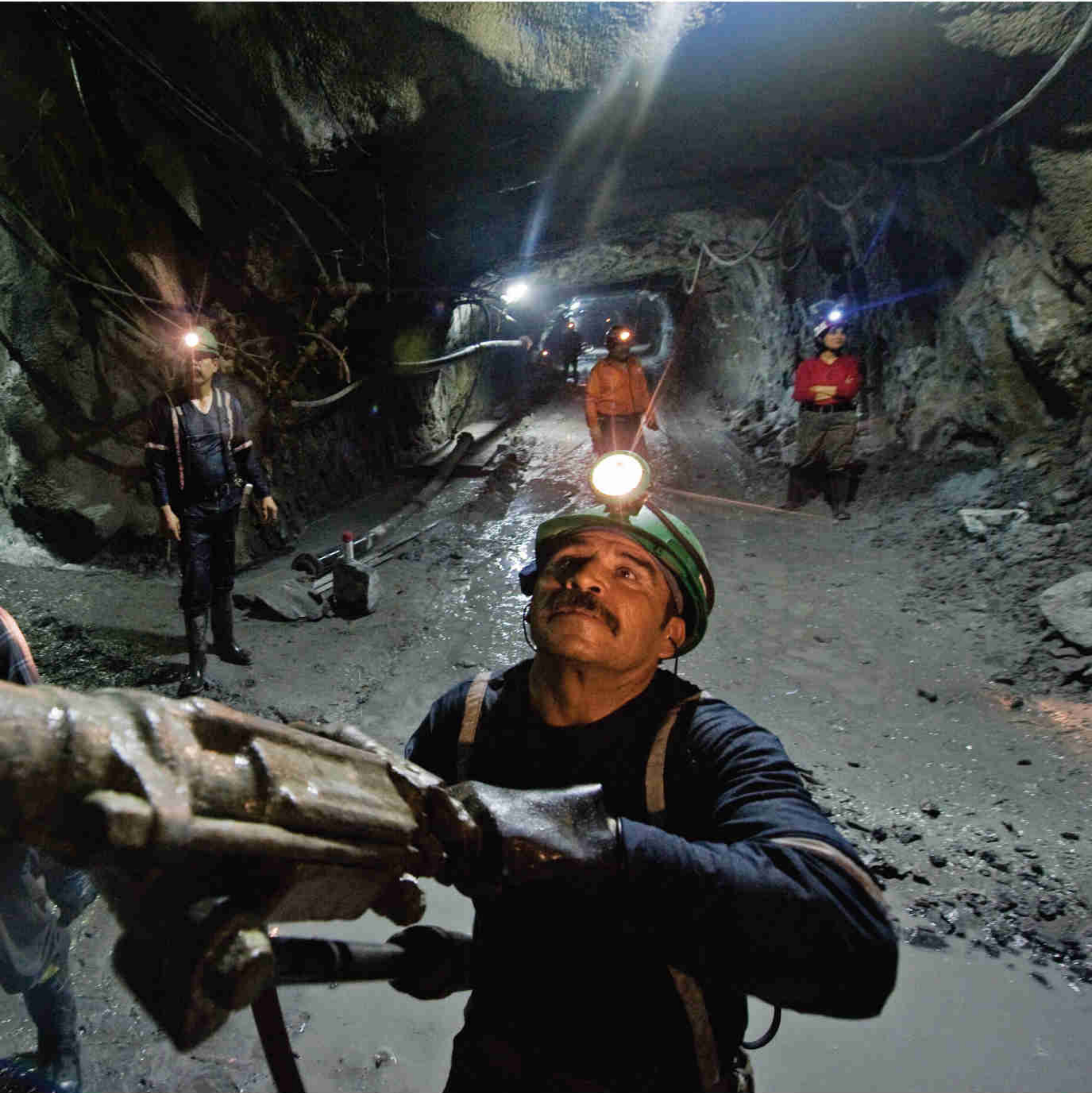
Chewing out space for cables and pipes, workers toil in the Naica mine, where excavations in 2000 led to the chance discovery of the giant crystals. Several other chambers bearing smaller crystals have been found in Naica, Mexico's most productive lead mine.
